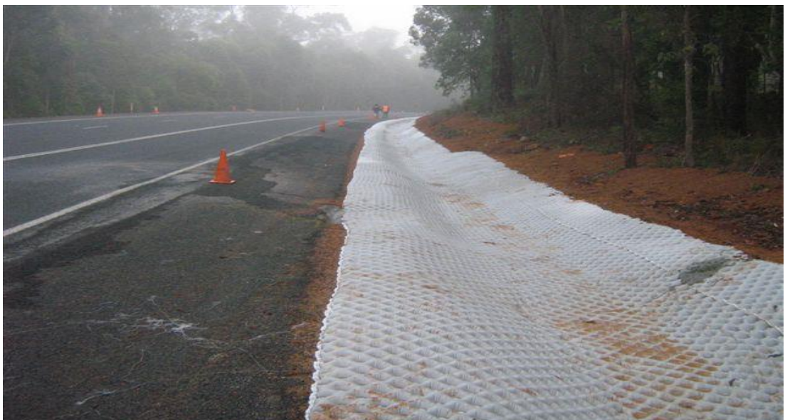
Use of grout filled mattress revetment systems for a roadside drain to prevent soil erosion.
